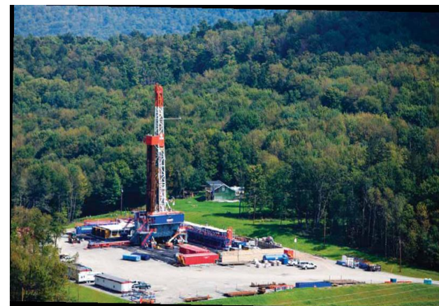
Fracking well site in Dimock, PA 1
